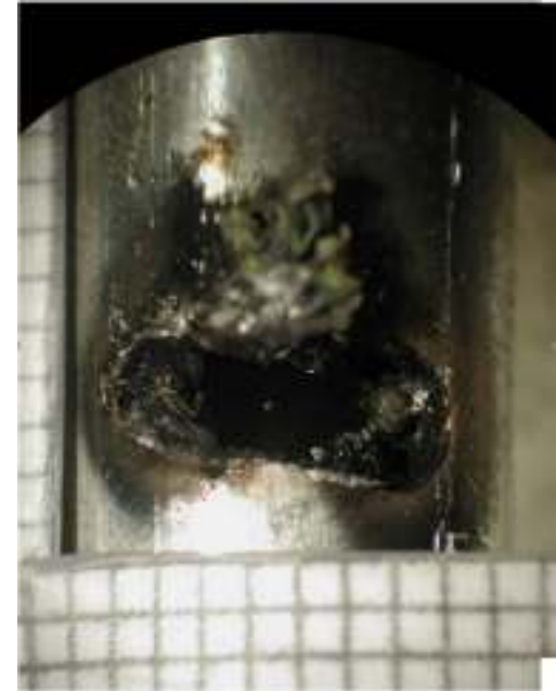
Example of arc damage to unpressurized tube
